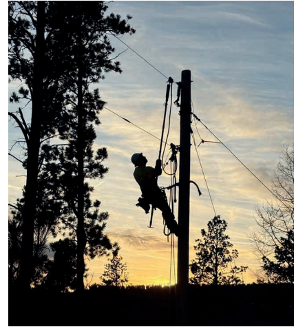
An assisting lineman from West River Electric Cooperative installs a ground on the line to be further worked on.
