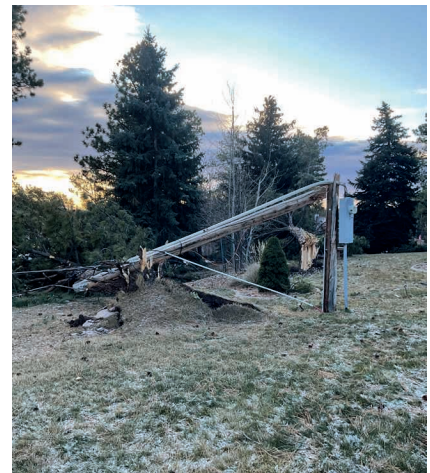
Damage from the storm not only affected poles, but also uprooted trees.
