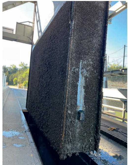
Zebra Mussels completely envelop Gavins Point Dam's water gates, adding up to an additional 30 tons of weight.
